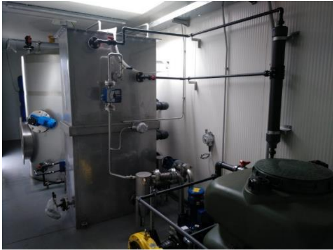
Anaerobic membrane bioreactor
